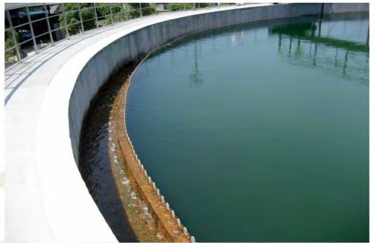
Effluent from sedimentation pond
