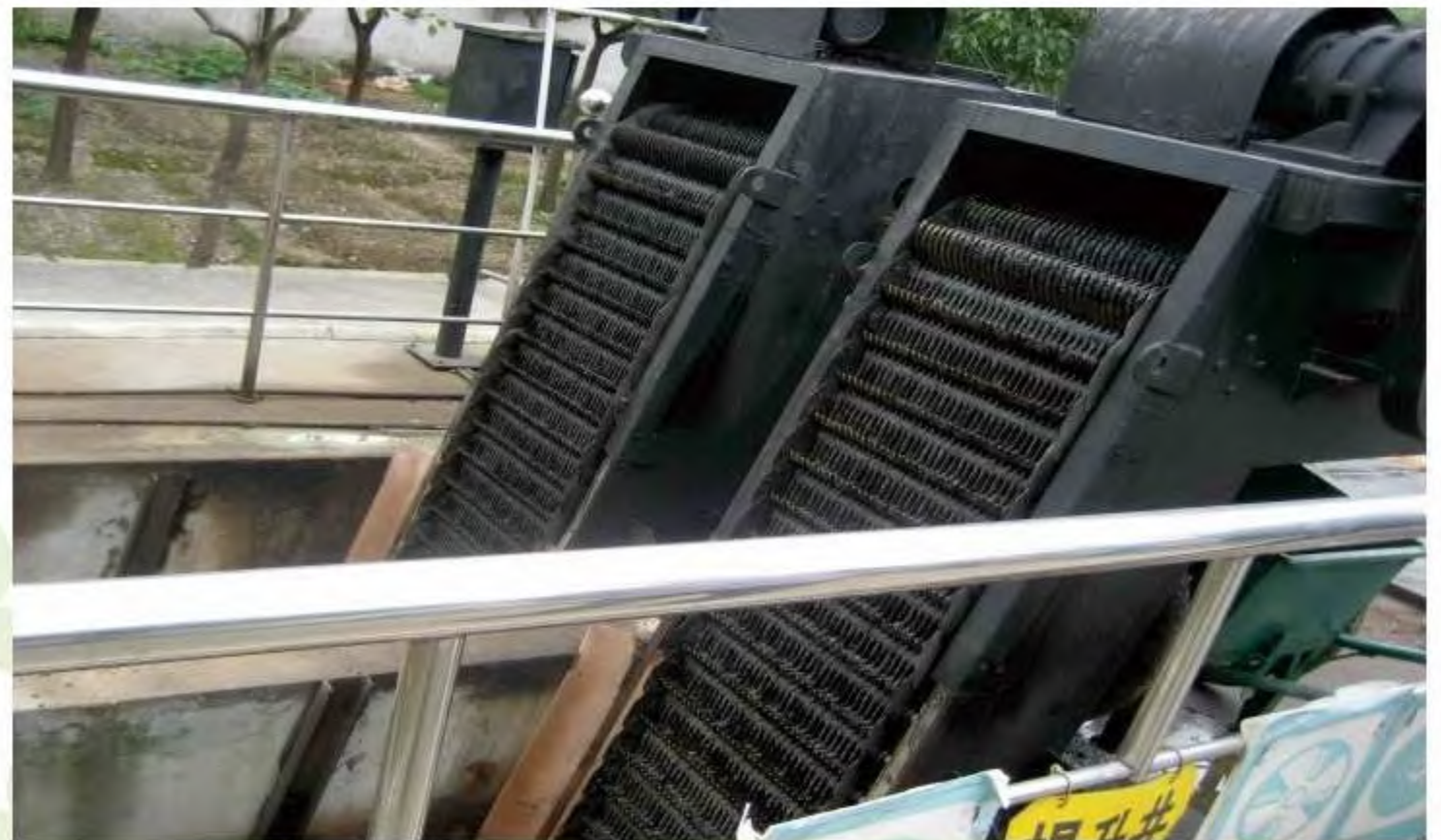
Pre-treatment by grit removal
